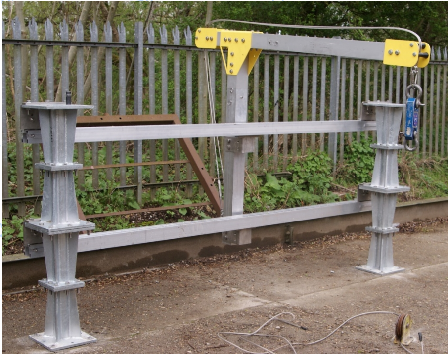
Figure 1 – Anchor rail described as “ERD.1500.1500 EdgeReil Davit” mounted on a stack of 4 davit bases
